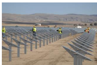
Topaz Project – California 550 MW
